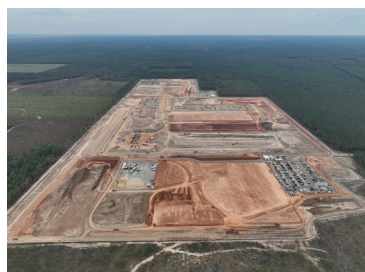
Data Center in north Louisiana
